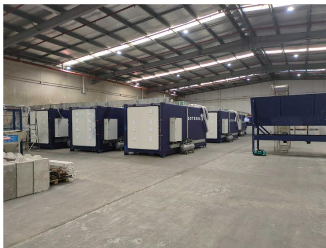
Figure 2 Goterra's insulated production systems (picture courtesy of Goterra)
